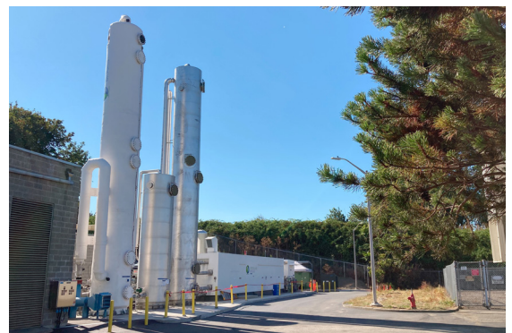
Cascade H 2 O installation
